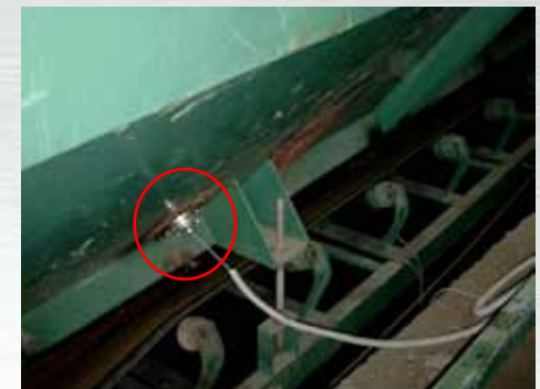
FSV in a wall of a weighing container
